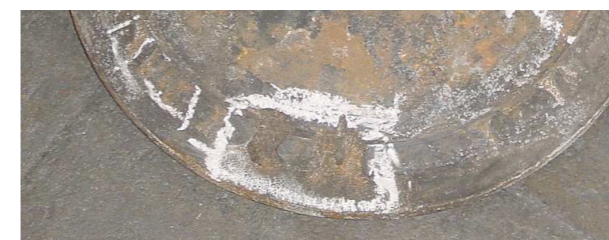
Figure 08: "Cobble stone corrosion" appearance of valve spindle failure through high-temperature corrosion (MC60 Standard-type)
